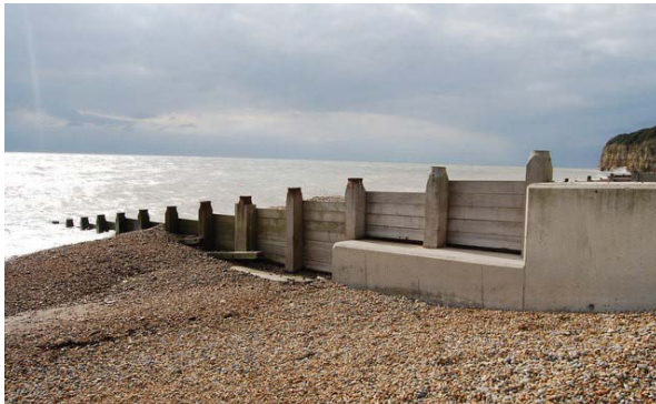
Example of hard engineering solutions, a concrete and wooden groyne, Photo Credit: Nigel Chadwick
